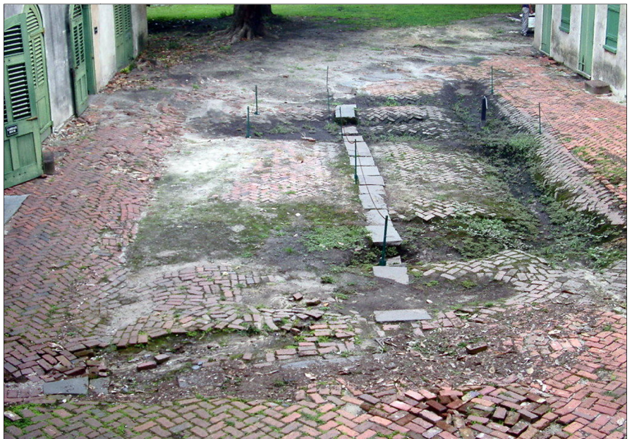
Regular depressions in the paved courtyard
