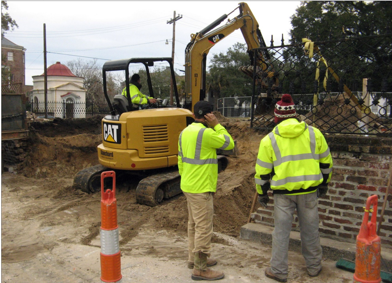
Excavation of the footprint for new stairs at Wragg Mall entrance on Meeting Street
