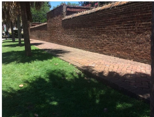
Figure 10. Photo of “dip” located in the projected path of Feature 15 (photo from the Post and Courier).
